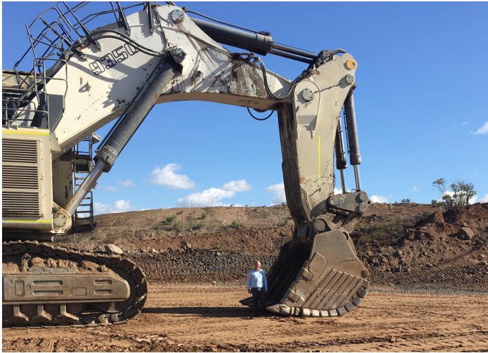
The mining excavator used to construct our composting pad was so big, they moved a hill in just one day
